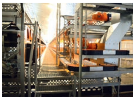
Inspection aisle in front of the first and second nest row
