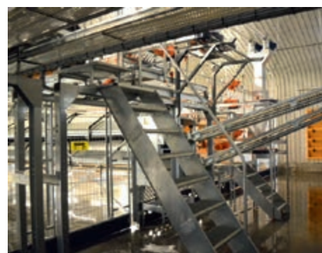
Stairs for the end sets make reaching the inspection aisles easy
