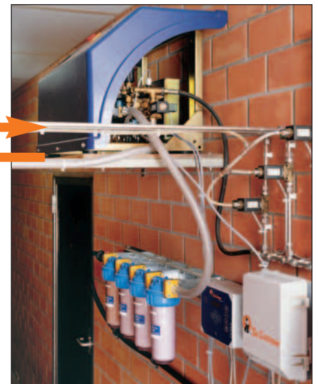
Central pump unit with 4-step filter
