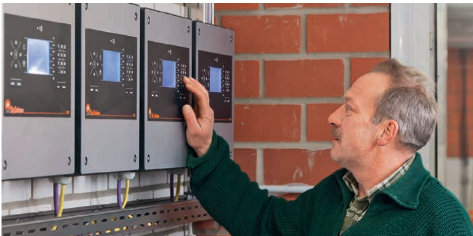
Each sorting scale TriSortpro is managed by a control unit, in this case installed in the service room
